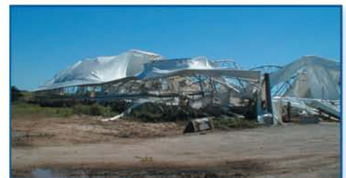
Even though the steel trusses of the buildings were twisted and crushed to the ground, the building held together. None of the 1450 cowherd were lost.
