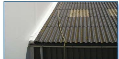
A fabric weather flap has been installed between the Cover-All and the metal clad building for water protection.
