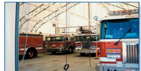
Mechanical components include radiant heating, electrical and extensive ventilation
