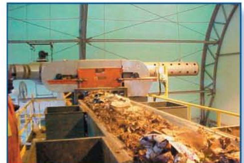
Sorting line and electro magnet remove large contaminants in receiving hall.
