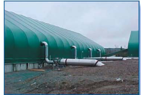
Bio-filters protect workers and control odor.
