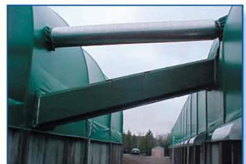
Enclosed conveyor transports sorted organics to compost halls.
