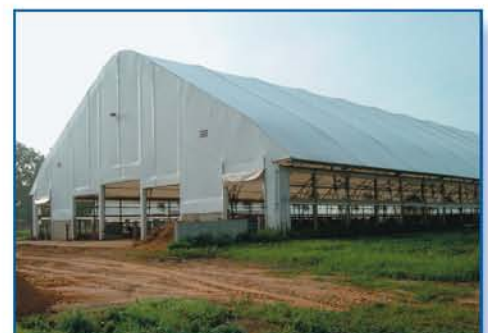
"We were able to design the barn to get all the natural ventilation we need," says Tim Hood.
