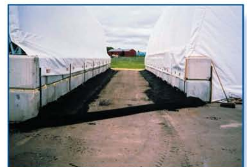
The lock-block foundation and asphalt pad ensure there is no harmful water run-off
