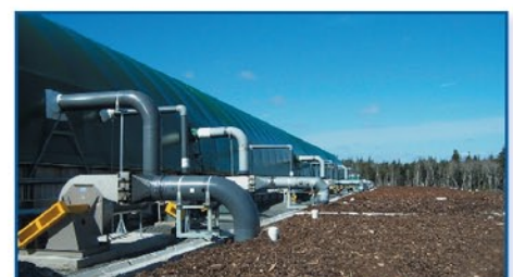
Exhausted air is filtered through an elaborate Bio Filter system to maintain negative air pressure, reduce indoor fog and control indoor air environment
