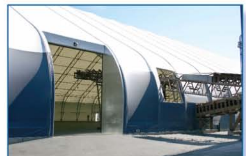
Three 16' wide by 20' high (4.8m x 6.0m) overhead doors were installed in the Cover-All® building.
