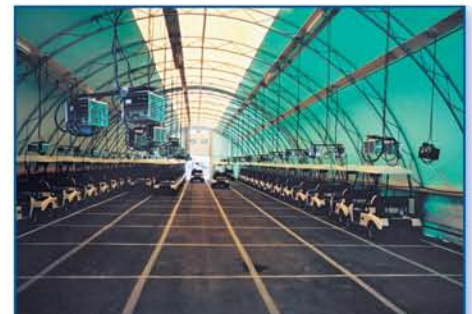
“At full capacity, we are able to hold 124 power carts inside with every cart having one electric charger,” says Burgart.
