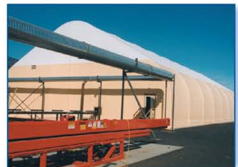
Installation of the new 12,800 square foot TITAN manufacturing facility took only four days
