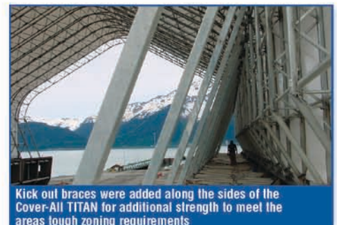
The massive dry dock facility is comprised of a 110' x 210' Cover-All TITAN mounted on a 55' x 220' steel foundation
