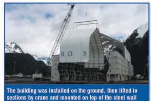
Kick out braces were added along the sides of the Cover-All TITAN for additional strength to meet the areas tough zoning requirements
