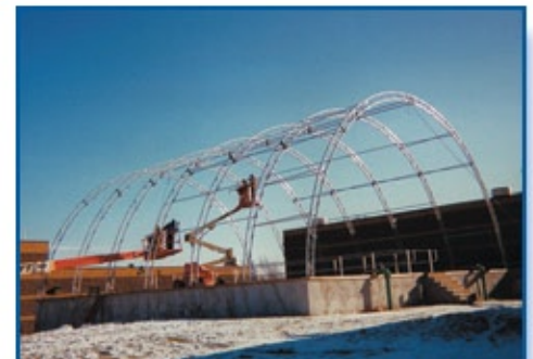
A crane lifted trusses into place while the tanks were still in use. A zoom boom was used to install cross purlins and to pull the fabric cover over the trusses.
