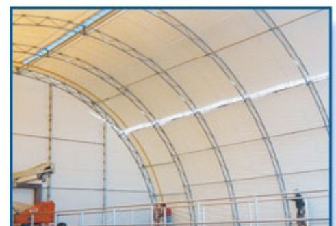
The six inch center ridge vent eliminates condensation problems and provides natural ventilation.
