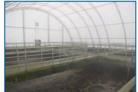
The Cover-All buildings were installed over the existing sludge tanks and designed with side accesses for installing equipment and cleaning the digesters.
